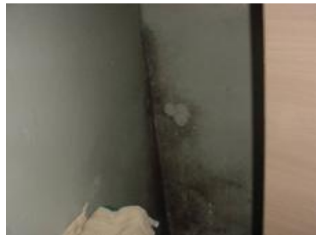
Mould from condensation in the corner of a bedroom
