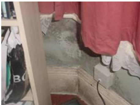
Mould from condensation to a bay wall
